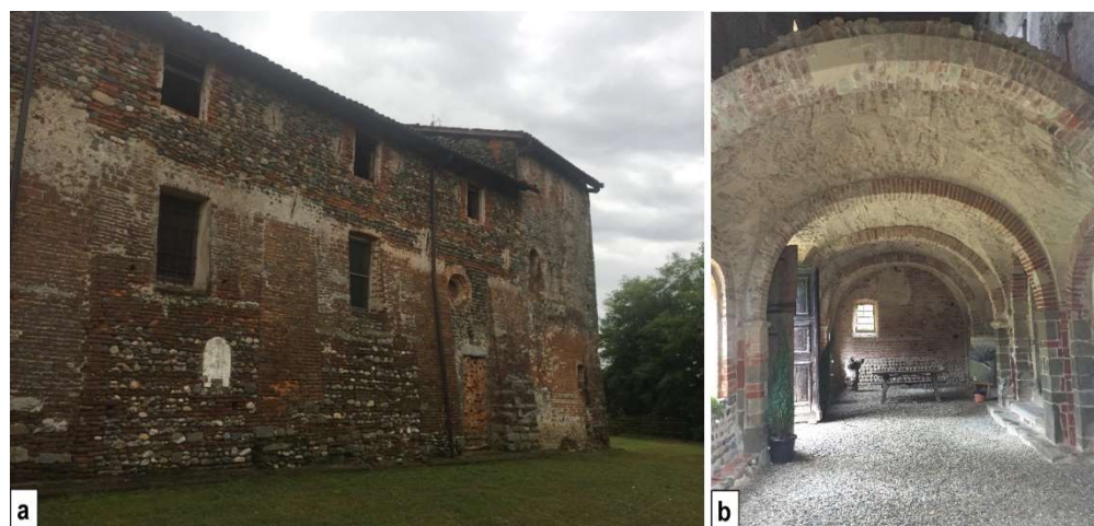
Figure 3.24: External (a.) and interior arcades (b.) of priory masonry of San Pietro at Castelletto Cervo (BI).
