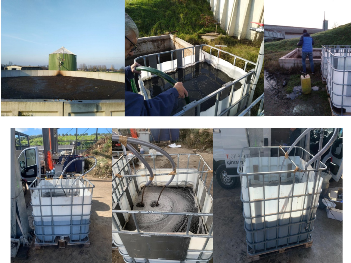
Figure 52: Scale-up industrial plant realization.
