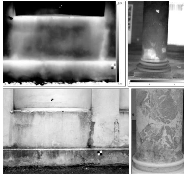
Figure 5.46. East façade (left), and main façade left column (right) anomalies were observed by thermographic imaging and principal component analysis of the multiband data (first components).
