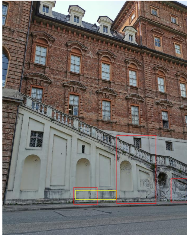
Figure 5.41. Castello del Valentino riverside (east) façade. The preliminary surveys are indicated in red and the detailed surveys in yellow color.
