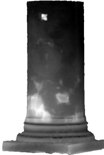
Figure 5.12. View of the final 3D thermal model of a column's base, where the position of restoration materials can be observed.
