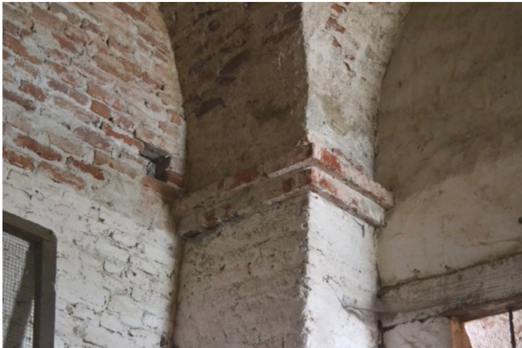
Figure 145. Detail of the walled pillar of the west wall. Picture taken from the additional camera created from the curtain west wall (Photo F. Diara)
