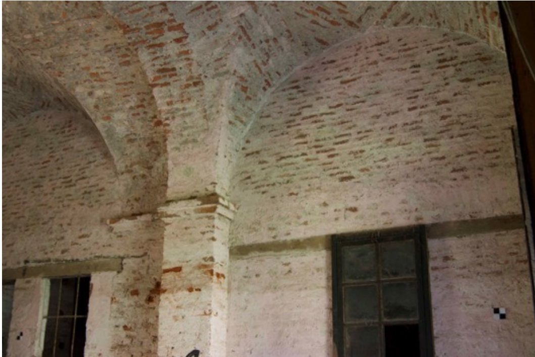
Figure 144. West wall of the refectory and detail on the walled pillar and the new vaulted system (Photo F. Diara)
