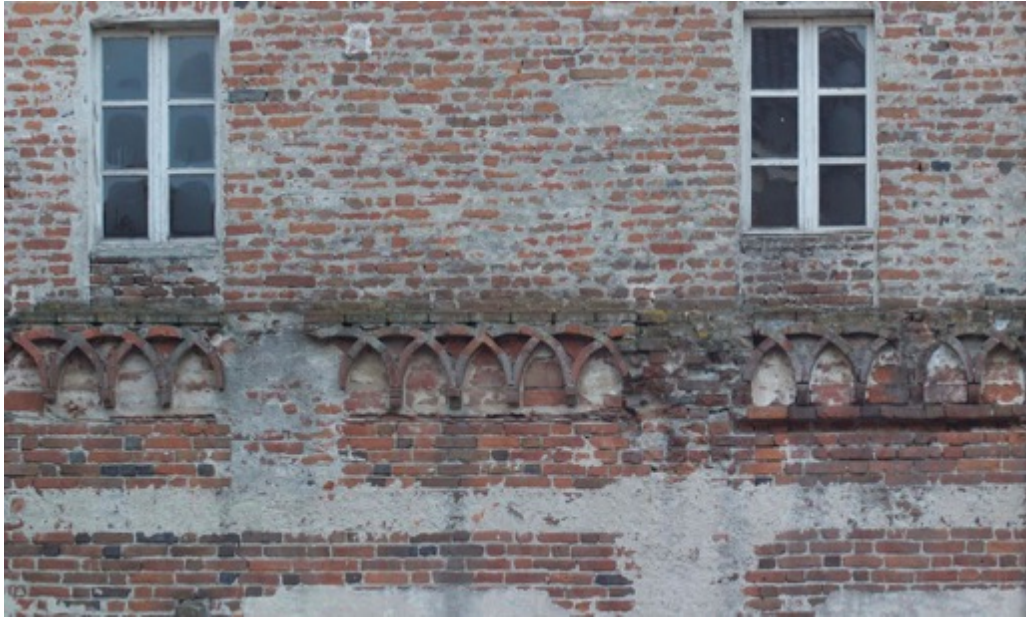
Figure 138. Suspended crossed arches on the south front of the cloister (the older height edge) (Photo F. Diara)
