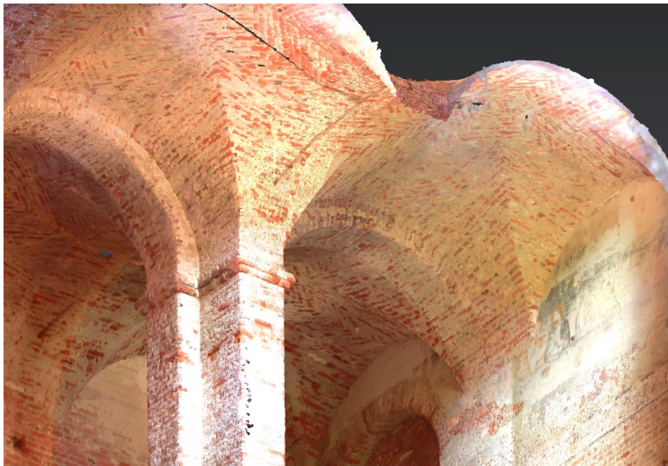
Figure 30. LiDAR point cloud of Staffarda refectory: detail of the intrados of the vaulted system (point cloud management by F. Diara)
