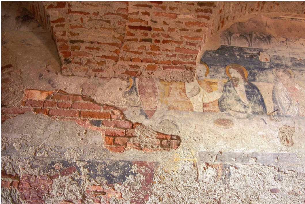
Figure 25. East wall of the refectory: detail of the Ultima Cena fresco, its preliminary plaster and on the left of picture evidence of the earlier plaster that shows an imitation of bricks (photo F. Diara)
