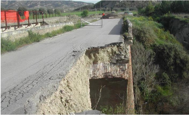
Figure 3. Bridge on SP 103: picture taken a few day after the collapse.
