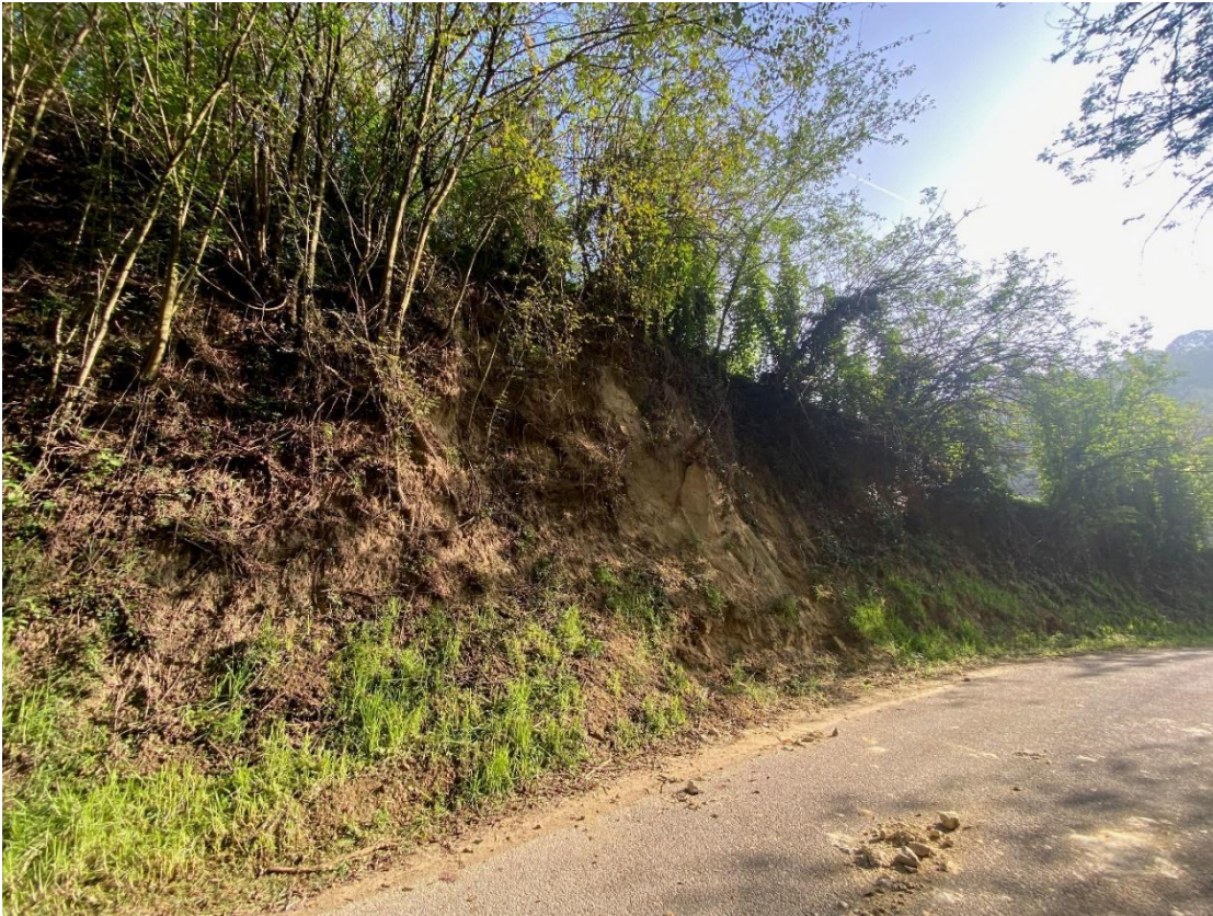
Figure 12 Wall subject to small-scale collapse in the Moncucco area.
