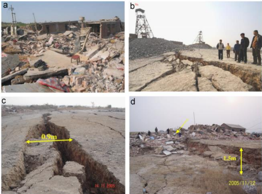
Figure 1.1 Damages produced by a large ground collapse occurred in Xingtai gypsum mines (China) in 2005: (a) collapse of surface buildings; (b) inclination and failure of surface land; (c) failure on surface land; (d) vertical dislocation through surface infrastructures (Wang et al. 2008)
