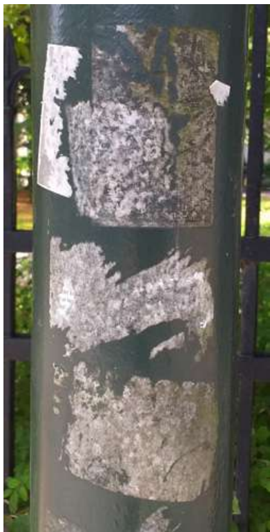
Figure 7: Sticker remnants on Lund's street signs columns.
