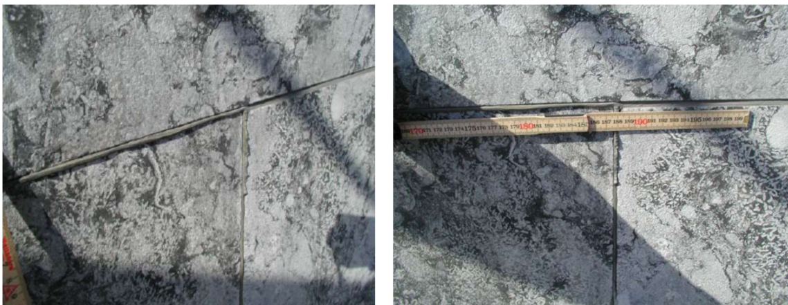
Figure 2.19 – Deformation in panels causing compaction of joint material (GELK et al, 2004)
