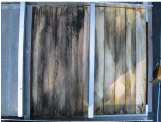
Figure: P6, Double layer set-up without edge sealing (opened): First decay in Poplar uncoated P6, Tannin glued left: lower side right: upper side
