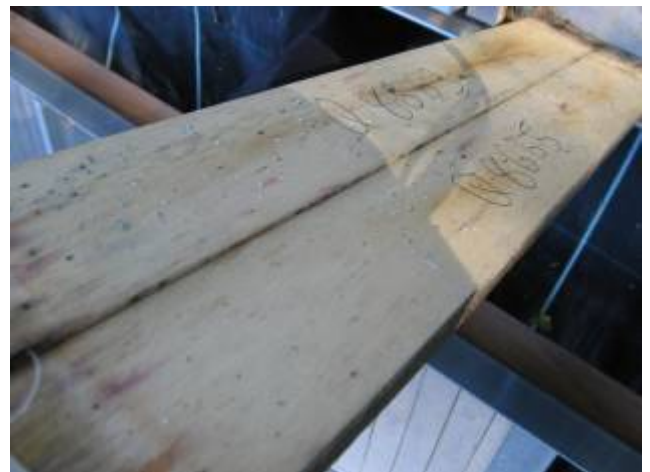
Figure: P12 , Poplar uncoated, MUF, P12: Moulds inside of double layer
