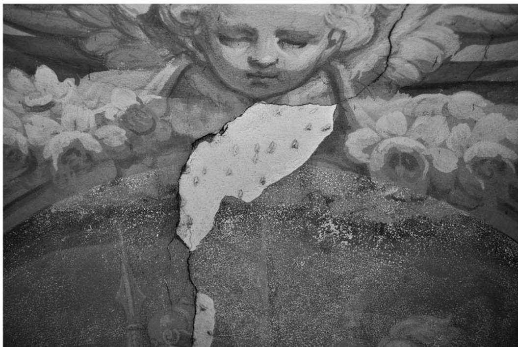
Figure 4. In the picture it is clearly observable the whitish surface of the mid '700 plaster, which was lately in mid '800 scaled with hammer to obtain a rough surface for a better adhesion of the new mortar and pictorial decoration. FOV 40 cm.
