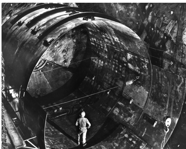
Fig. 3. Construction of the tank used in the solar neutrino experiment in the Homestake gold mine (Courtesy: Brookhaven National Laboratory).
