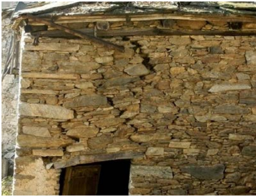
Fig. 3. The main crack pattern is caused by a differential soil settlement.
