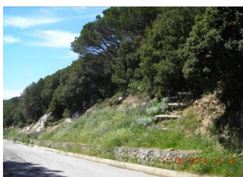
Vegetated Crib wall in the Mediterranean area- Slopes Sardegna, Italy. P. Cornellini AIPIN EFIB
