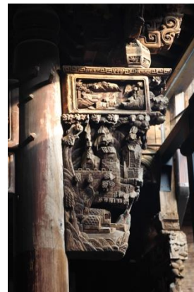
Pic. 6 Large amounts of wood material and fine wood carvings inner the buildings
