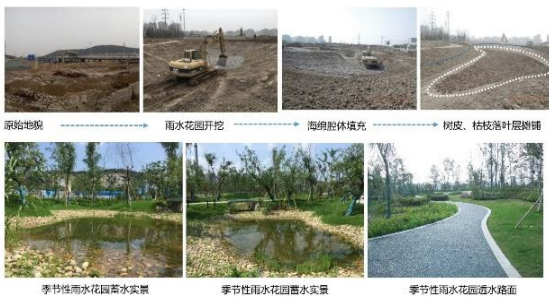
Fig.13. Han Shan road node sponge green space construction process and completion effect.
