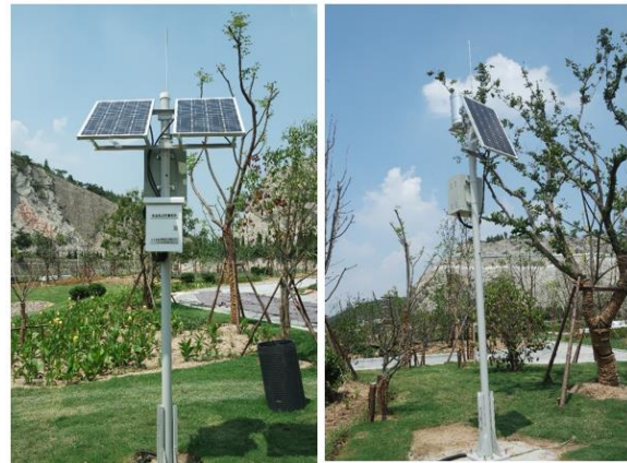
Fig.14. Water environment measurement and control system of Xiang Wang Road.
