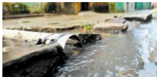
Fig. 2. Sewage disposal in the urban drainage network– Fortaleza City – Brazil.
