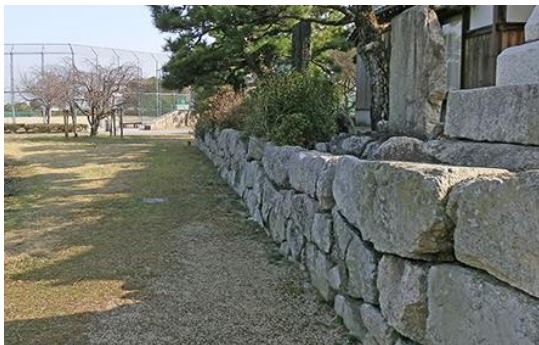
Fig. 2. Image of a masonry retaining wall supporting the site of a temple
