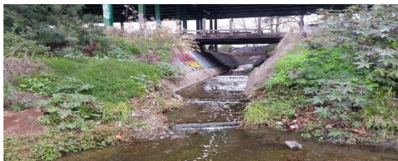
Fig. 2. The creek as flood control culvert courses under the grey infrastructure of freeways and railroad tracks.
