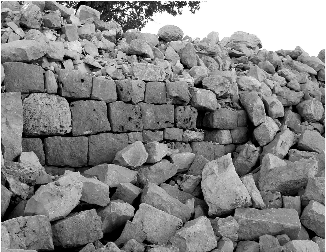
Fig. 13. Bilevah. Decayed wall in undressed blocks of masonry (© Centro Scavi Torino and ICAR)
