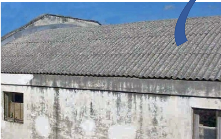
anthropogenic sources i.e. roofs containing asbestos
