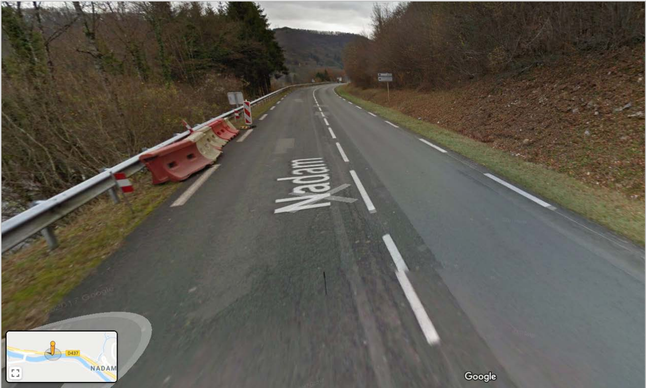
Figure 8 - View of the asset at stake – Road RD437 at the bottom of zone A.
