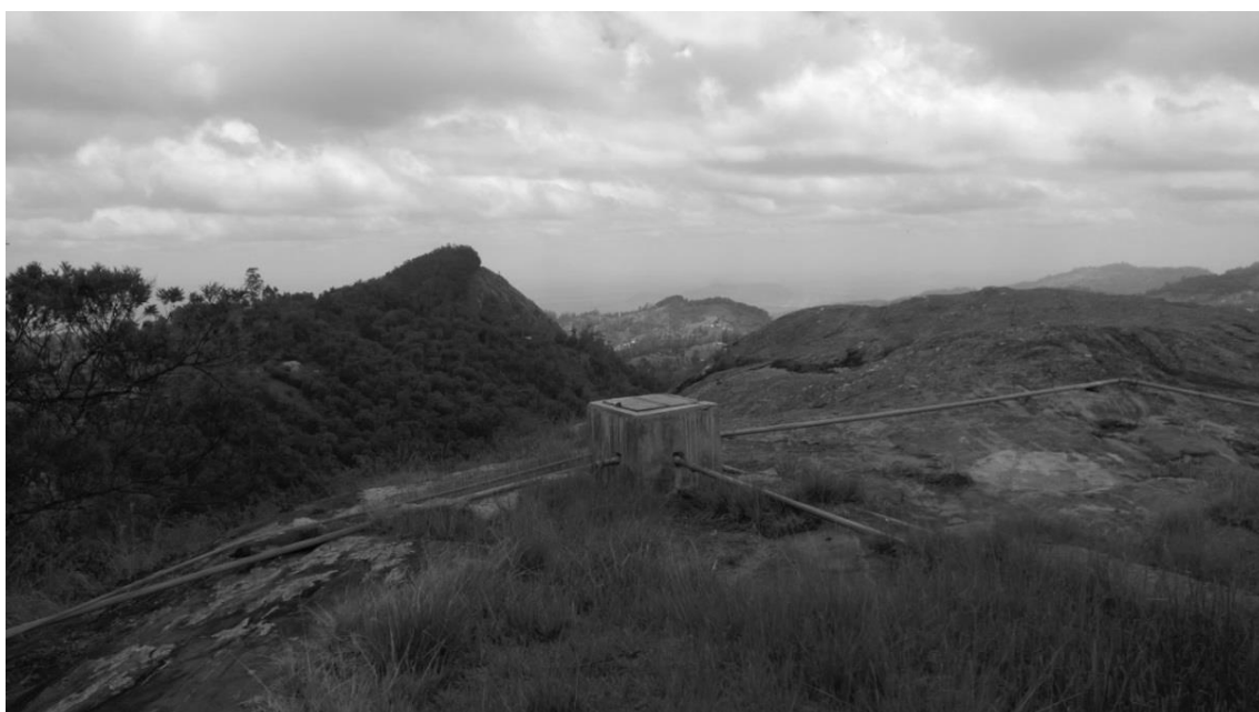
Figure 15. In many cases, the maintenance of the water structures falls on the community members themselves, who might not have the technical knowledge or funds to repair the water infrastructure. These pipes on the top of Kiangungu hill were leaking in February 2013 and thus a village nearby had been without water supply for three weeks (Kivivuori 2013)
