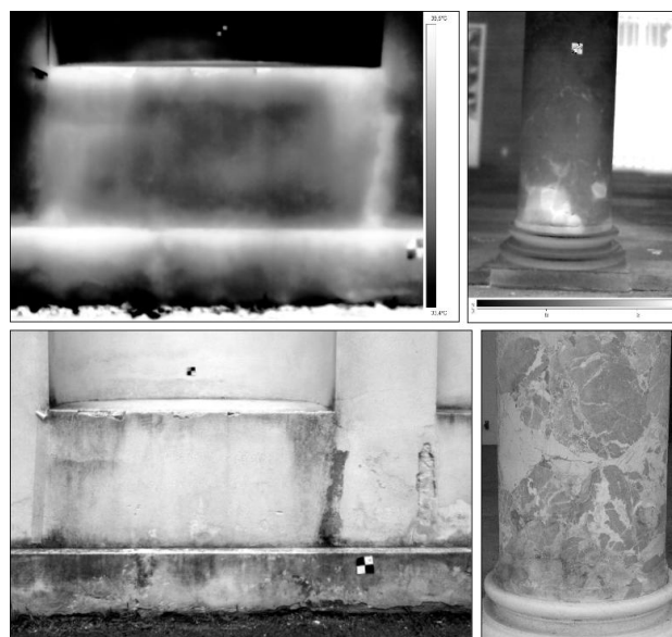
Figure 7. East façade (left), and main façade left column (right) anomalies observed by thermographic imaging and principal component analysis of the multiband data (first components).
