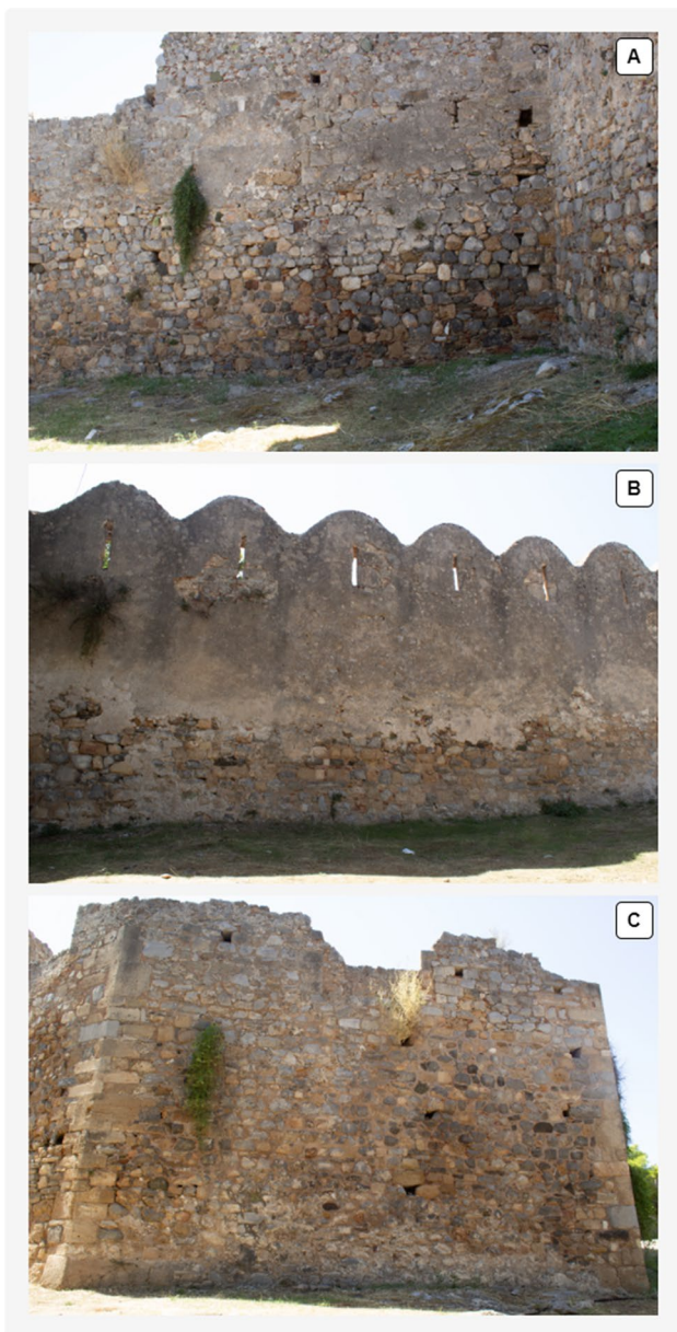
Fig. 3 Fort of Karababa north side, façades selected for evaluating the mapping methodology; from top to bottom: A (westernmost), B , and C (easternmost)
