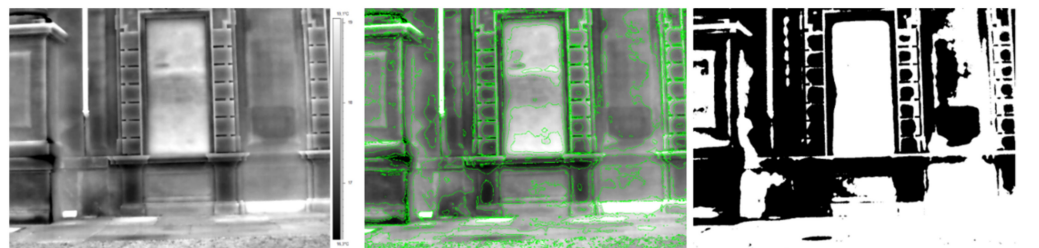
Figure 5. Thermographic image elaboration for Turin's Castello del Valentino (Italy): (left) original thermogram; (center) thermal contours (every 0.5\text{ }^{\circ}\text{C} ); (right) thresholded thermogram (at 17.7\text{ }^{\circ}\text{C} ).
