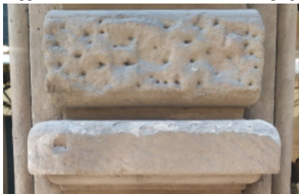
Fig. 1: The Bossage under study with evident damage due to flaking and exfoliation. Samples are taken from areas already decoached without further damage to the artwork
