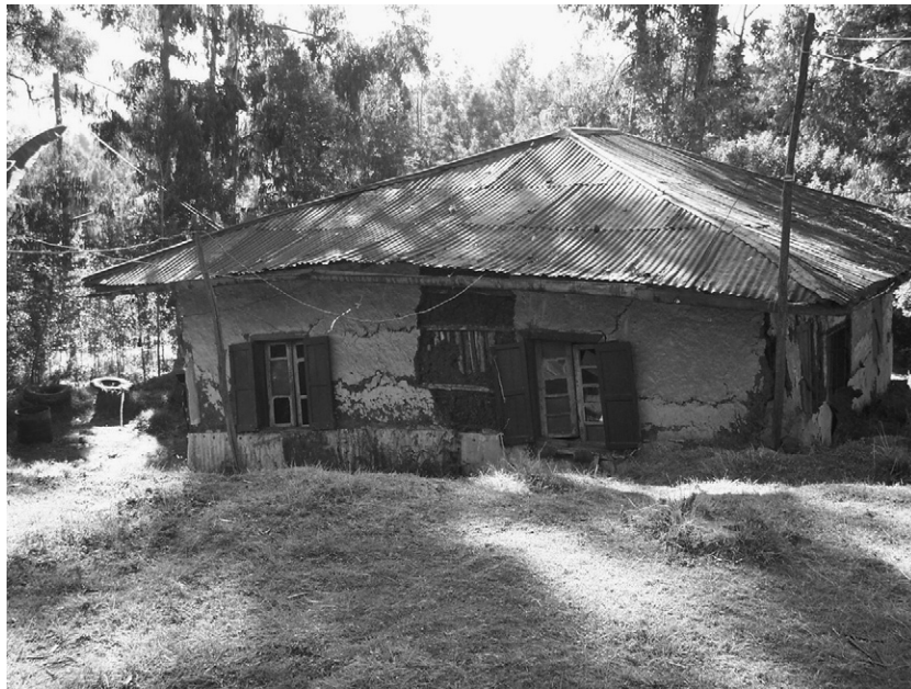
Fig. 11. House tilted by a slow moving landslide since 1994.
