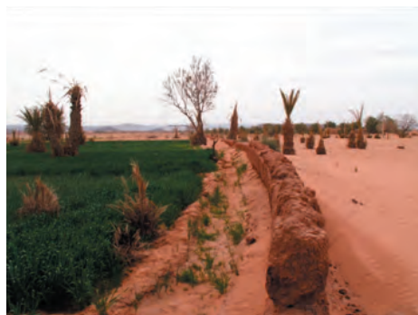
Figure 14. Protection wall against the siltation of the palm grove in Ait Ben Omar (Ferkla).
