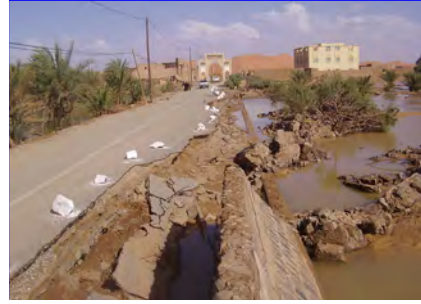
Figure 3. State of the road after a flood, at the entrance of Merzouga.
